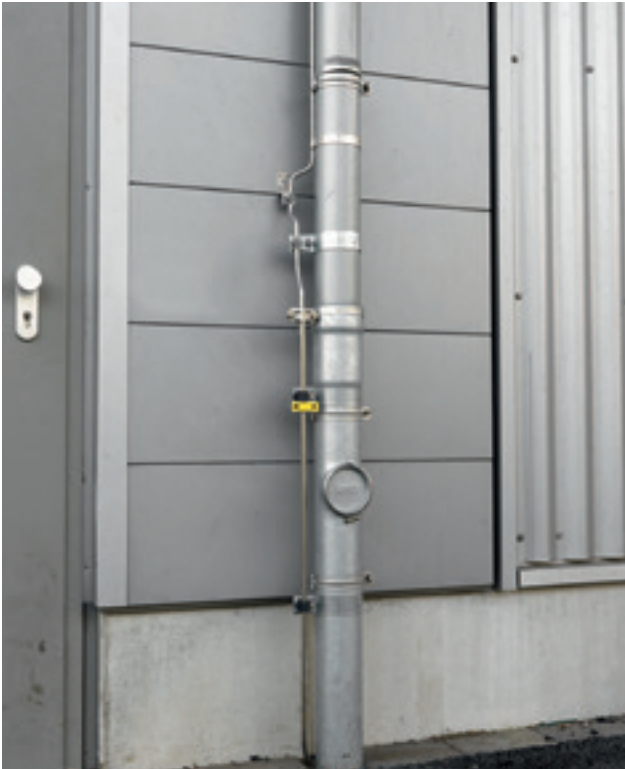
Lightning protection conductor on a rainwater downpipe
